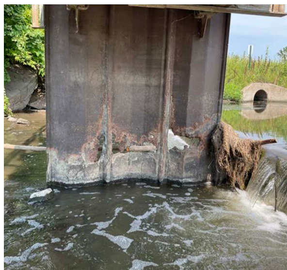
Deterioration at Bridge over Beckwith Rd
